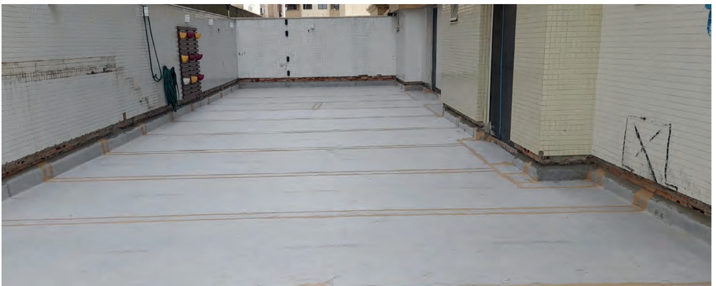
Waterproofing of 700 m 2 with ECODRY120 on all its outdoor walkable terraces. Condo in Itapema. Brazil.
