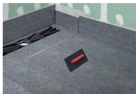
15. Check that the membrane is extended and use a trowel to remove the air that may have been generated.
