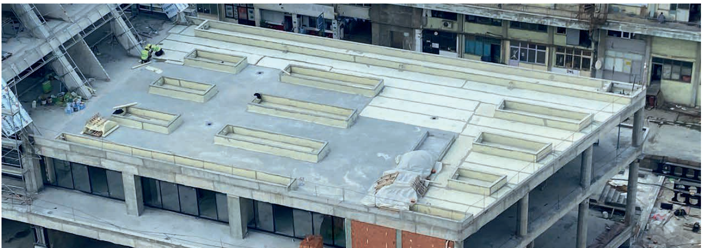
Waterproofing of 20.000 m 2 of DRY120 in all its outdoor walkable terraces. ISTMALL ISTANBUL. Building for offices, university and shopping centre. Istanbul. Turkey.
