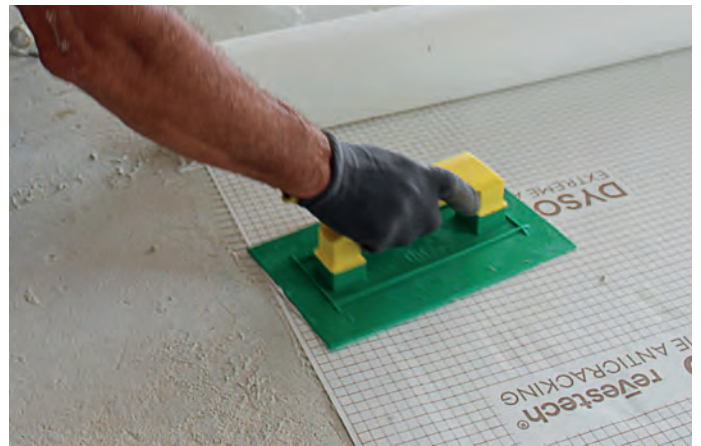
4. Press the DYSO smembrane hard on the structure with the help of a plastic trowel making sure to eliminate all possible air bubbles.
