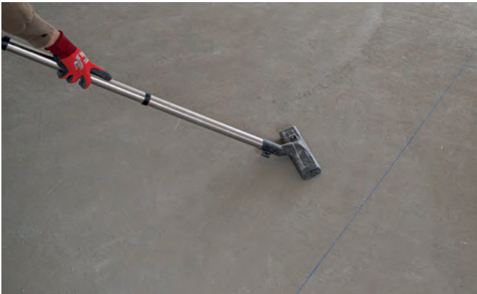
1. Check the stability of the structure and clean the surface. The structure must be clean of any element that may difficult the adhesion of the membrane.
