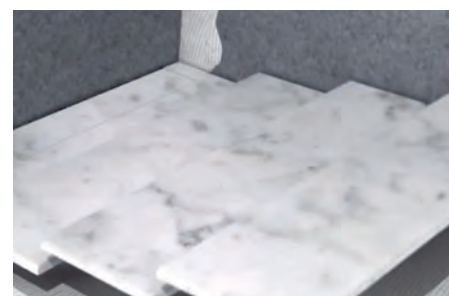
19. Proceed to cover the tray with tiles, starting from the eaves and always using the LINEAR/SUMI LEVEL as a guide.
