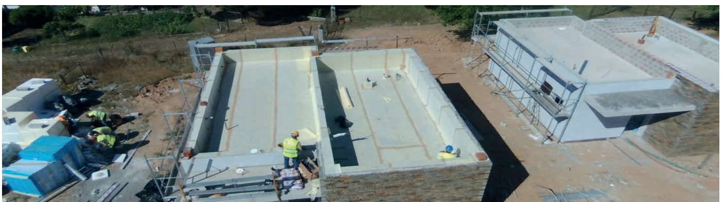
Waterproofing of roofs with DRY80 . CARE HOME IN LENSTISCAIS. Castelo Branco. Portugal.
